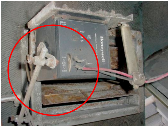
Small ventilation damper showing signs of damper and linkage corrosion.
