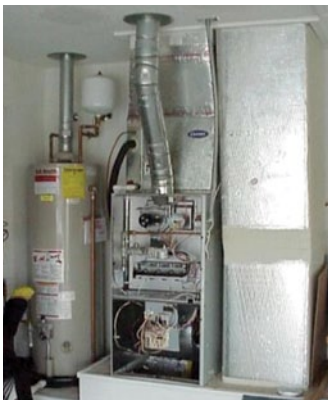
Gas furnace with panel removed. Cabinet and return duct leakage can interfere with natural draft appliances such as the gas water heater at left.
