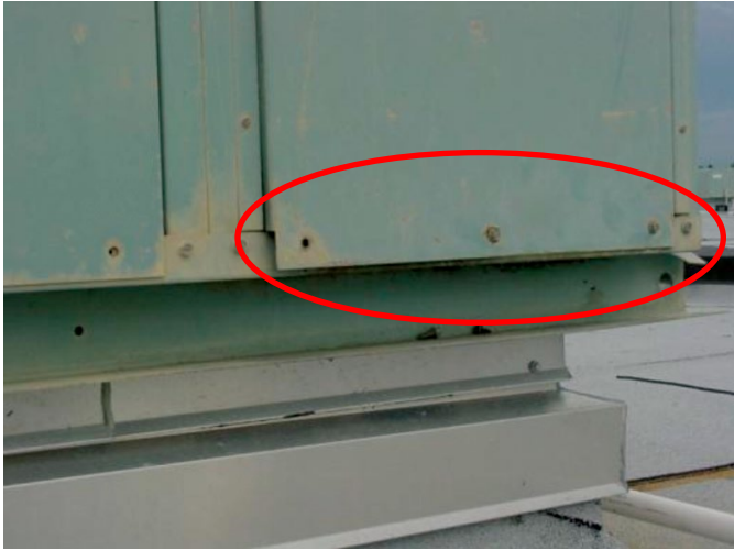
Roof top package unit leakage through loose panels.
