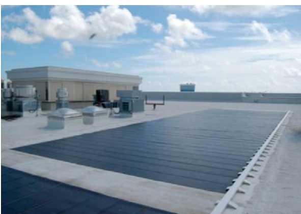
Thin film modules mounted on a flat roof. This flat-roof type is generally less efficient and requires more roof area than a sloped system.
