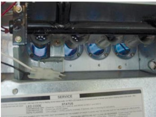
Light blue flames indicate clean efficient combustion.
