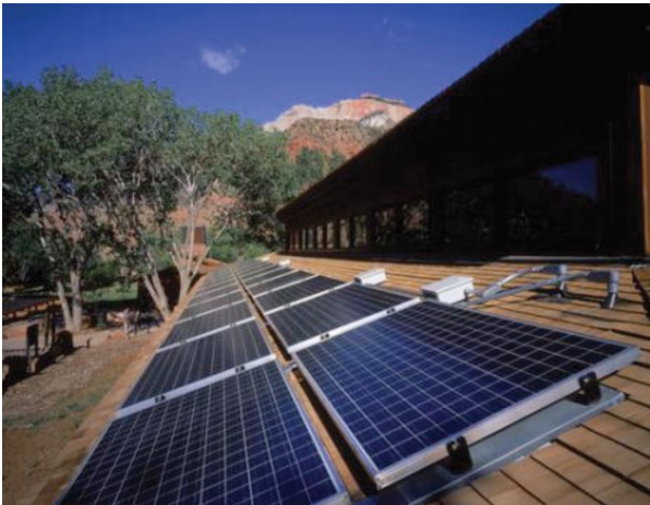
Crystalline modules mounted on a sloped roof. Source: Florida Solar Energy Center
