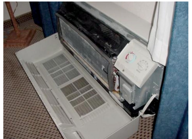
PTAC unit was not tilted toward the drain correctly and water spilled from condensate pan onto carpet below.
