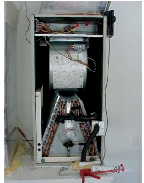
Inside view of AHU with blower above evaporator coil. Electric heat element is located above the blower.
