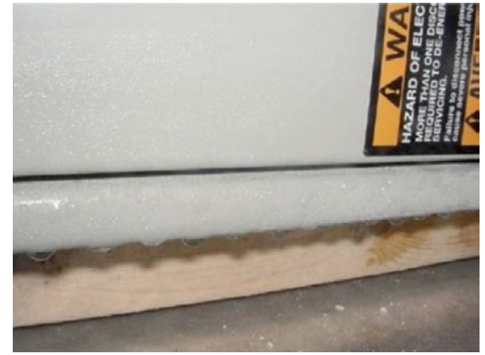
Condensation at bottom of air handler caused by wet interior insulation, rendering the insulation useless.
